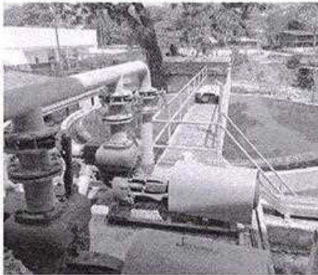
500 KLD STP at Kozhikode medical College
